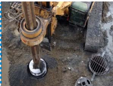
Bored Tension Pile: 35,000 m, Ø 1000 mm piles to the maximum depth of 15 m.
