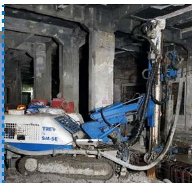
Underpinning micropiles: 2,000 m, Ø 250 mm micropiles to the maximum depth of 13 m.
