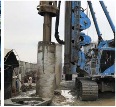
Secant piles: 7,000 m 2 , Ø 1000 mm piles to the maximum depth of 30 m.
