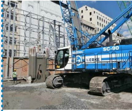
Diaphragm wall (Mechanical Grab): 18,000 m 2 , 1000 mm thick panels to the maximum depth of 35 m.
