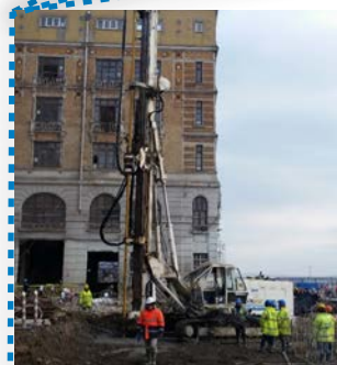
Jet Grouting bottom plug: 45,000 m 3 , Ø 2000 mm columns to the max depth of 29 m.
