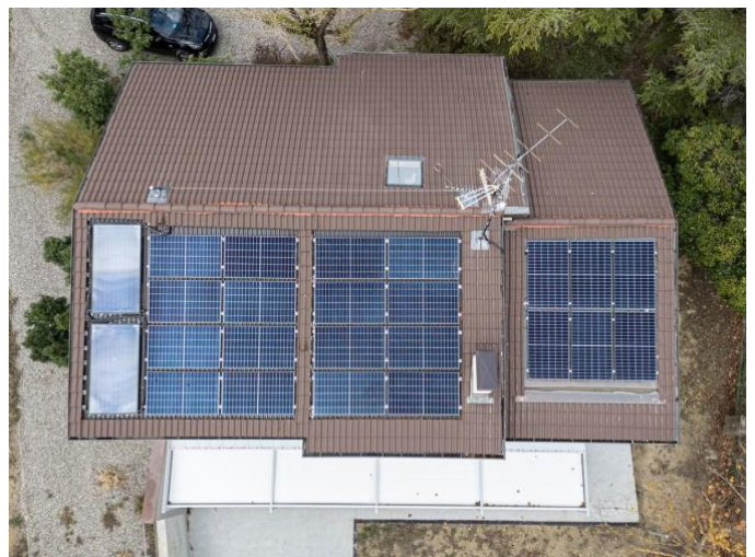
Aerial view — full roof PV + solar thermal installation
