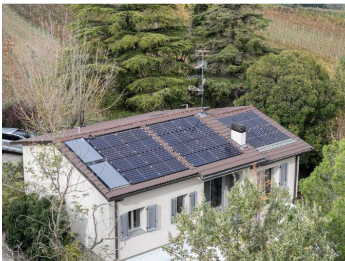
Residential villa — PV + solar thermal system, Imola area
