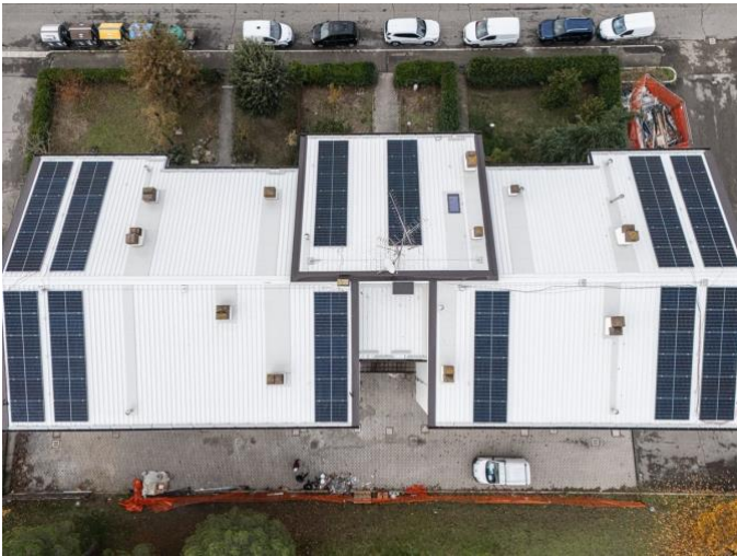
Industrial building — large-scale rooftop PV system
