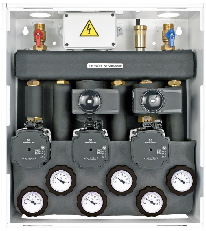
Photo with pumps 7 m pumps and servomotors NVM08 *
