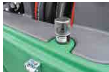
Monitoraggio intercapedine. Leak detector.
