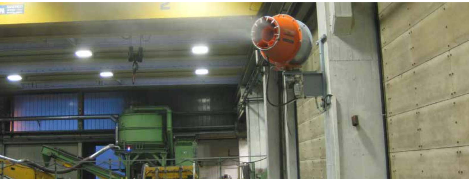
Diffused emission inside waste treatment plant - fixed Big Fogger Plus
