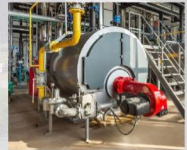
Steam Boilers high / low pressure
