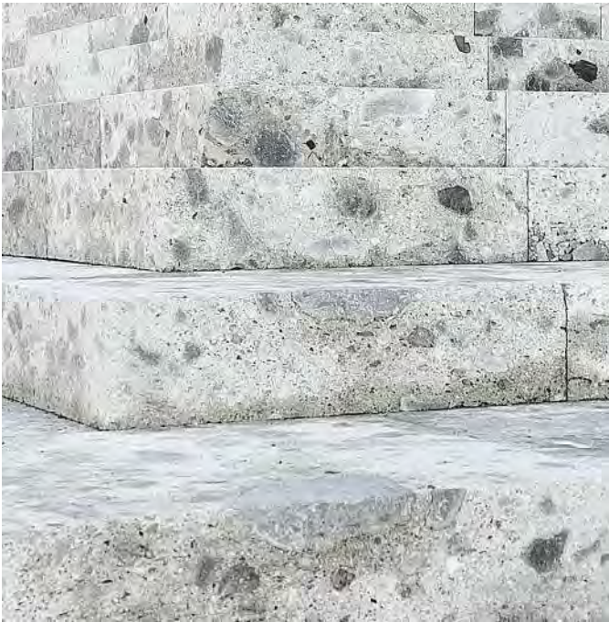
Pilgrim house – JXXIII Sotto il Monte Giovanni XXIII (BG) Detail of the staircase made of Ceppo di Gré stone
