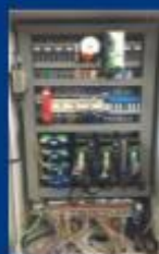
ELECTRIC PANEL COD. 027 0E
